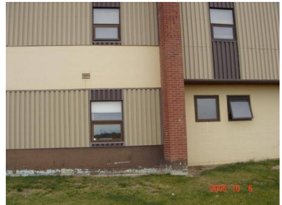
Damaged building finish due to lack of drainage
