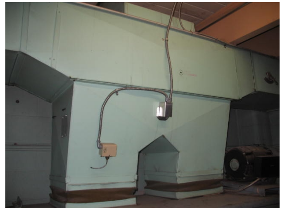
Unit Serving Gymnasium
