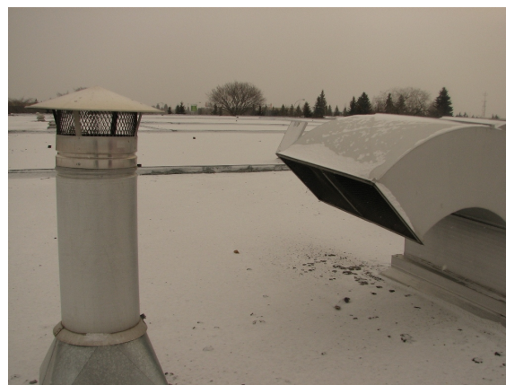
Proximity of Vent serving DWH to F/A intake.
