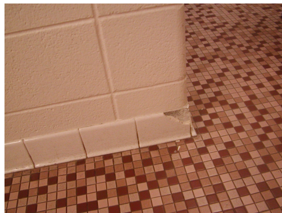
Damaged tile in boys washroom #22
