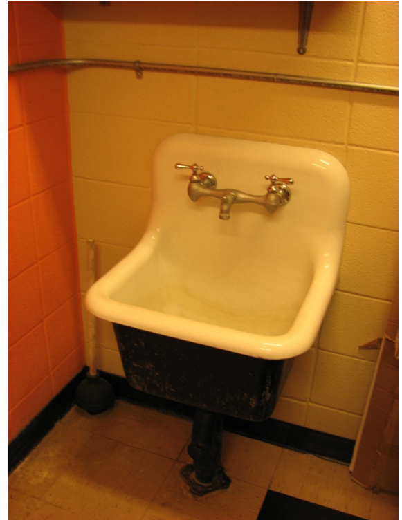
Wall hung mop sink that does not comply with the current Building Code.
