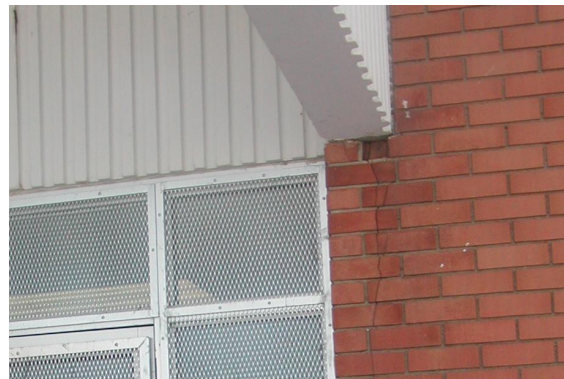
Stress crack at brick/tee at rear entrance.
