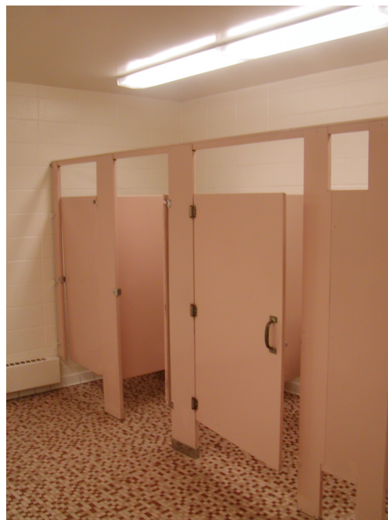
Toilet partitions in girls washroom #23
