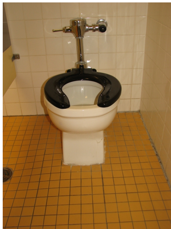
Water Closet is cracked.
