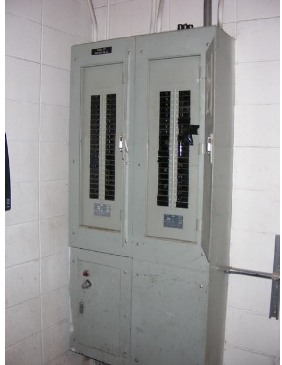
Aged electrical branch circuit panels.
