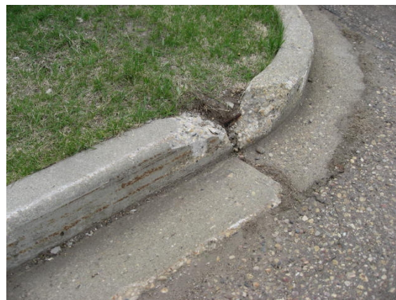
Damaged roadway curbs observed in several isolated areas.
