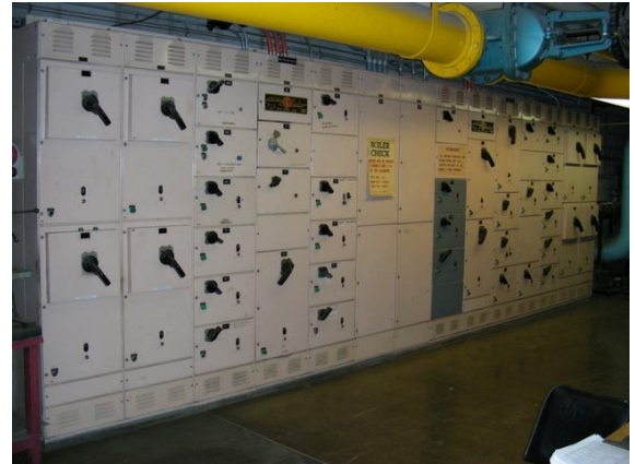
Aged MCC #3 and MCC #4
