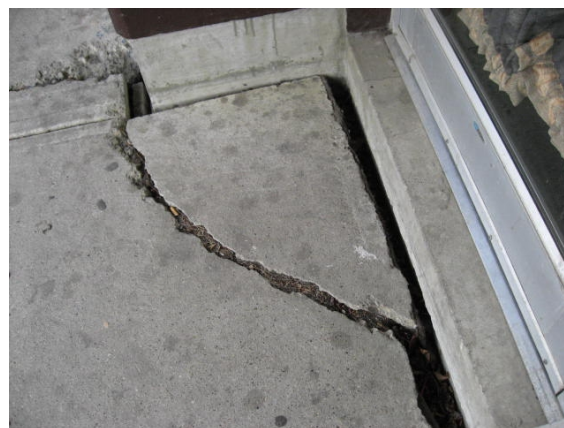
Settlement of concrete observed in several locations around the school.
