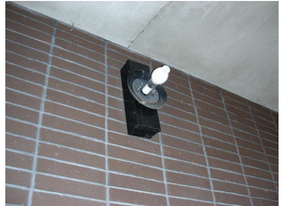
Damaged globe type fixture
