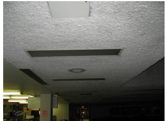
Sprayed textured ceiling in the cafeteria.
