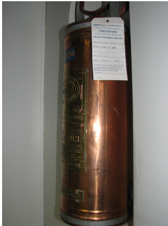
1951 original Pump Tank Fire extinguishers.
