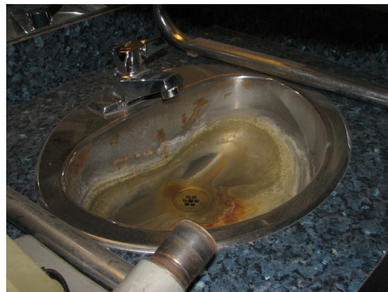
Rust present in lavatories, suggest that the water lines are rusted.
