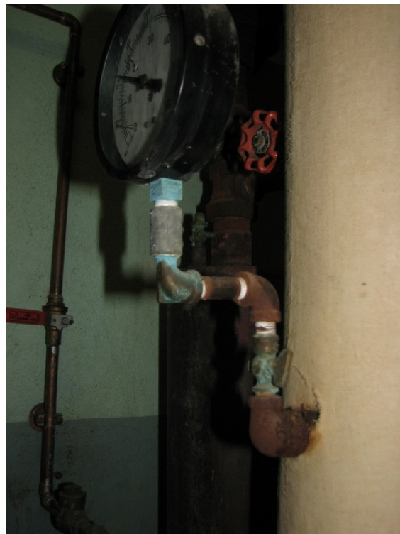
The following pictures show the condition of the Heating system in the school. All the components are corroded, rusted, show signs of age, and are a sign of imminent system failure.
