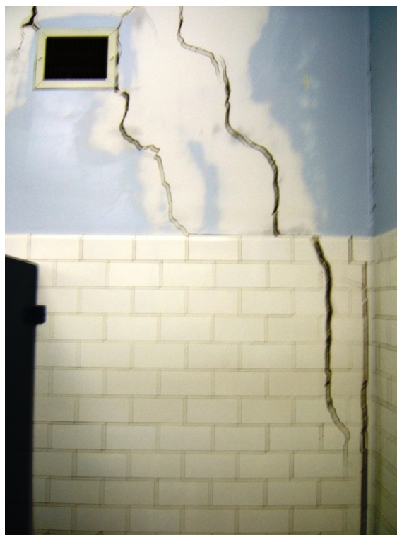
Wall crack in staff wash room of 1952 section.
