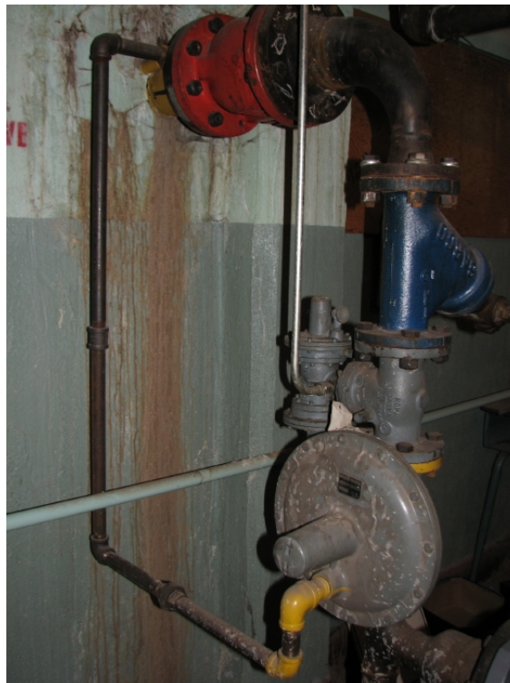
Rust and corrosion on main gas line.
