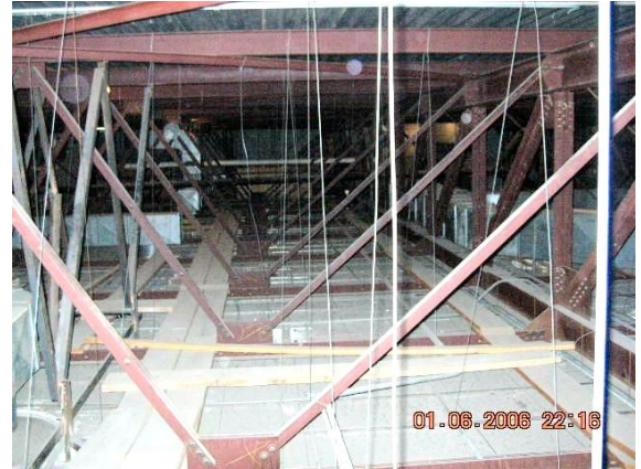
Catwalks in large Gymnasium truss spaces - loosely laid planks are unsafe.
