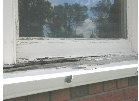
Typical deterioration of wood window frames.
