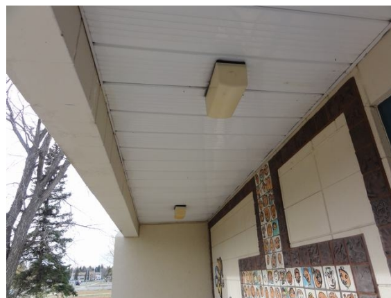
Incandescent lighting fixtures in soffit.
