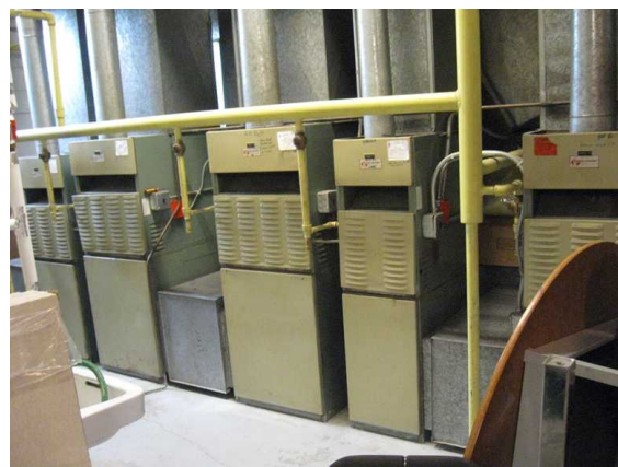
Typical Flame-Master furnaces in Mechanical Room
