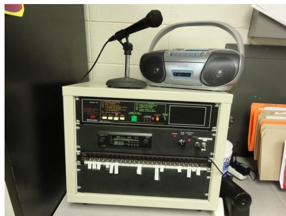
Bogen MCP-35A P.A. System in general office.
