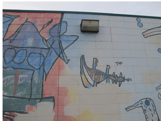
Structural movement between mortar joints on exterior east wall
