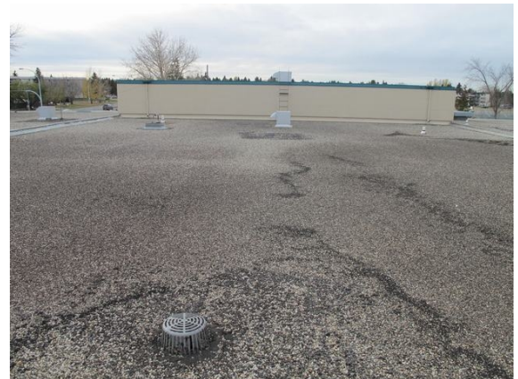
Several blisters and evidence of ponding throughout.
