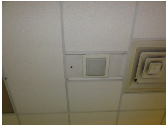
Ceiling mounted emergency lighting unit.
