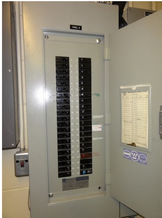
Westinghouse 120/208V branch circuit panel (1973).
