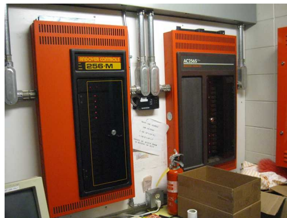
Andover main control panel in Mechanical Room
