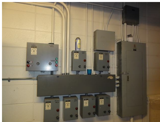
Westinghouse motor starters in mechanical room.
