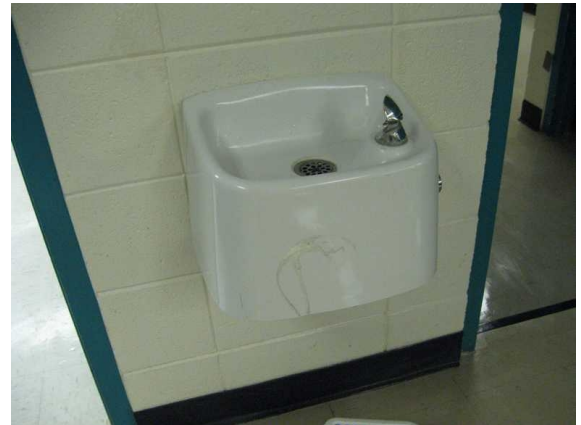
Drinking fountain with crack
