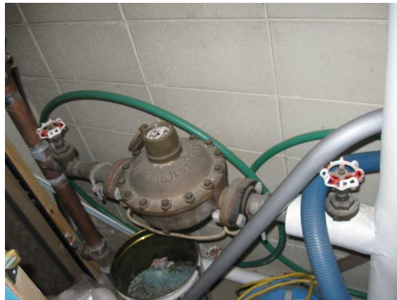
Domestic water main without backflow preventor
