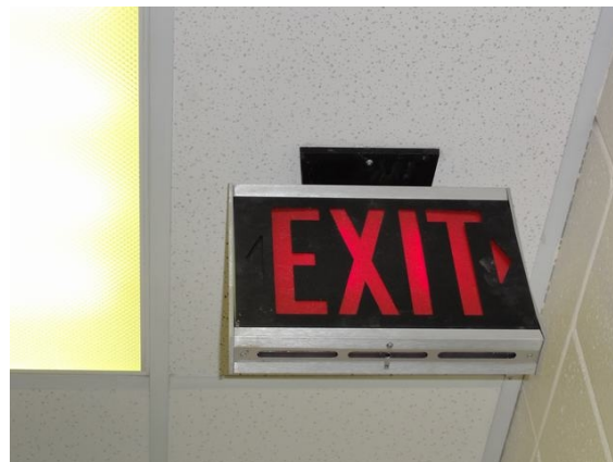
Exit sign in corridor.
