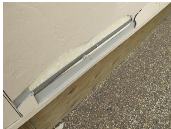
Damaged exterior stucco panel - South Elevation
