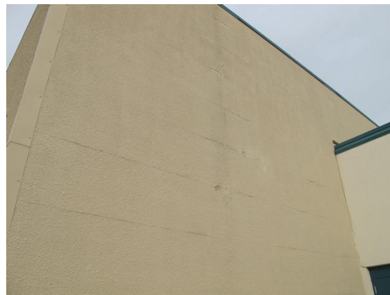
Cracks observed on the south elevation of the gymnasium wall.
