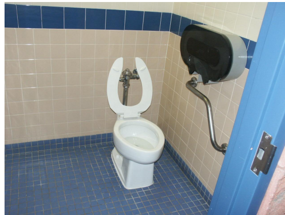
BFA cubicle missing grab bar over toilet.
