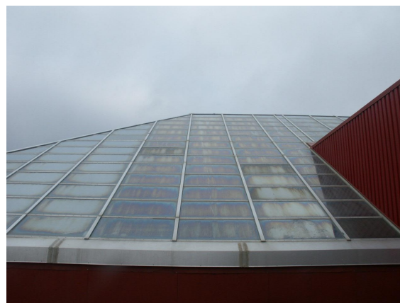
Oily slick on glazing related to caulking failure.
