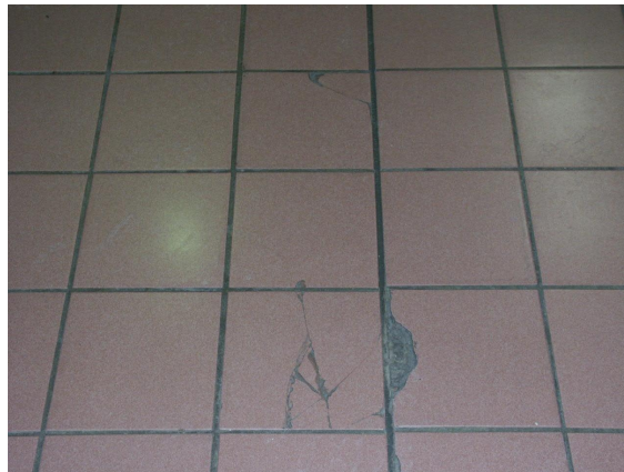
Cracked and damaged floor tiles in streets.
