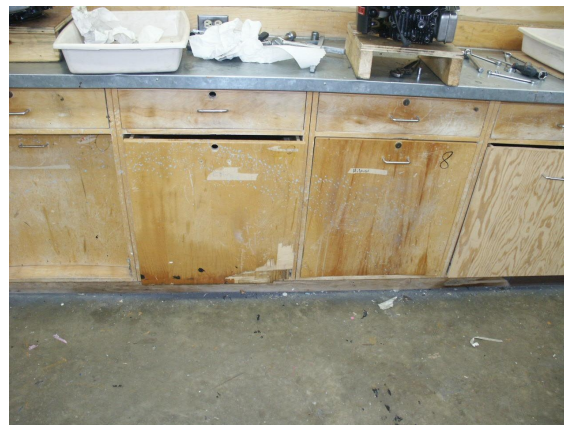
Stained and damaged casework.
