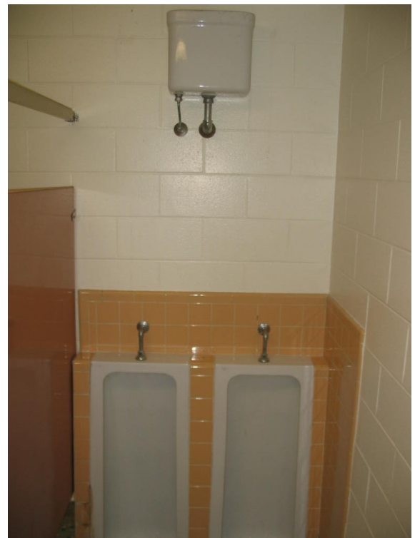
Flush tank urinals.
