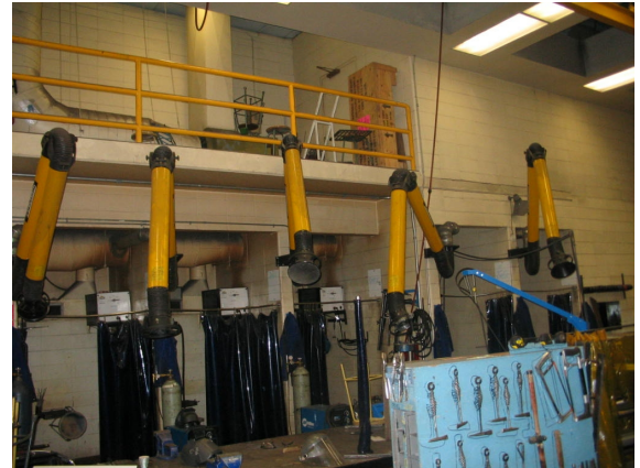
Flexible Extraction Arms in the Welding Area.
