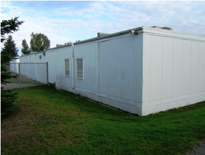
Partial view of portable units
