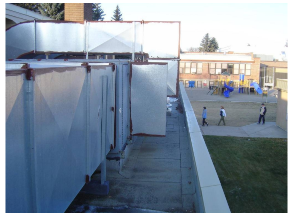
Service limitations at roof parapet for AHU-4.
