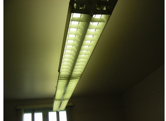
Aged louvered T12 fluorescent fixtures.
