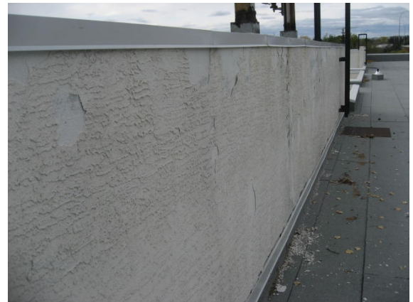
Deteriorated cement plaster finish on firewall - Roof Level
