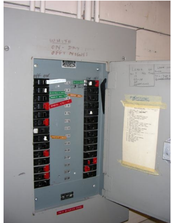
Aged branch circuit panel in main electrical room.
