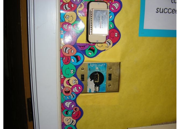
Aged 120V lighting switches.
