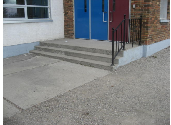
Cracked stairs at north-west entrance.
