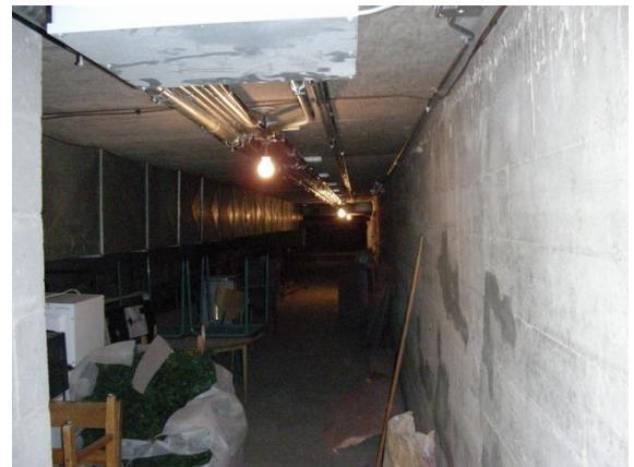
Incandescent lighting in service tunnel.
