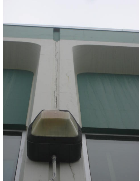
Caulk joint failure at precast connections.
