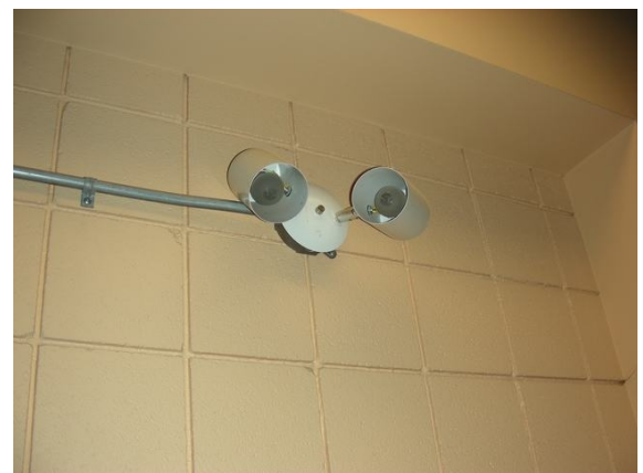
Incandescent emergency lighting heads.
