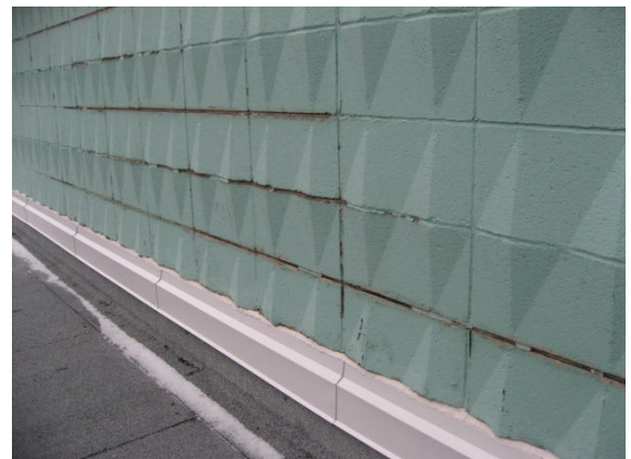
Deteriorated paint finish on concrete block walls
