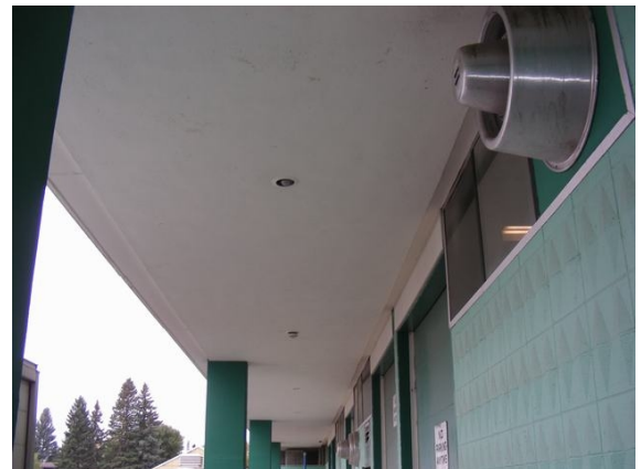
Exterior recessed incandescent lighting in canopy.
