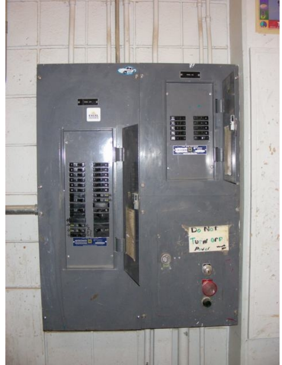
Aged Square D panel in shop area.
