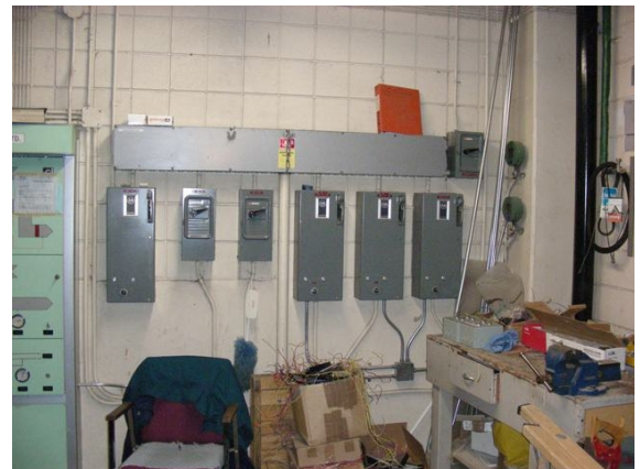
Allen Bradley motor starters.
