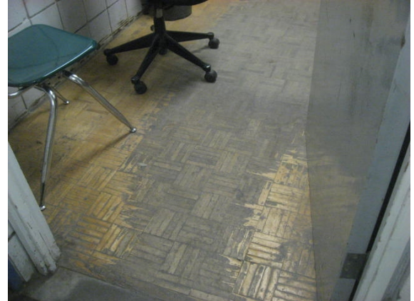
Deteriorated floor finish in the building construction shop area.
