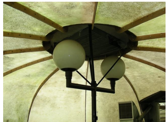
Incandescent pole mounted lighting in greenhouse.
