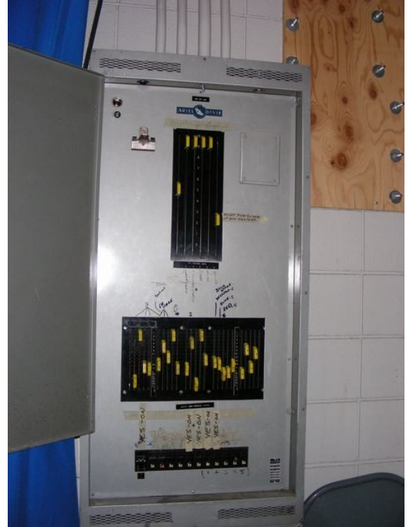
Obsolete Ariel Davis dimming system.
