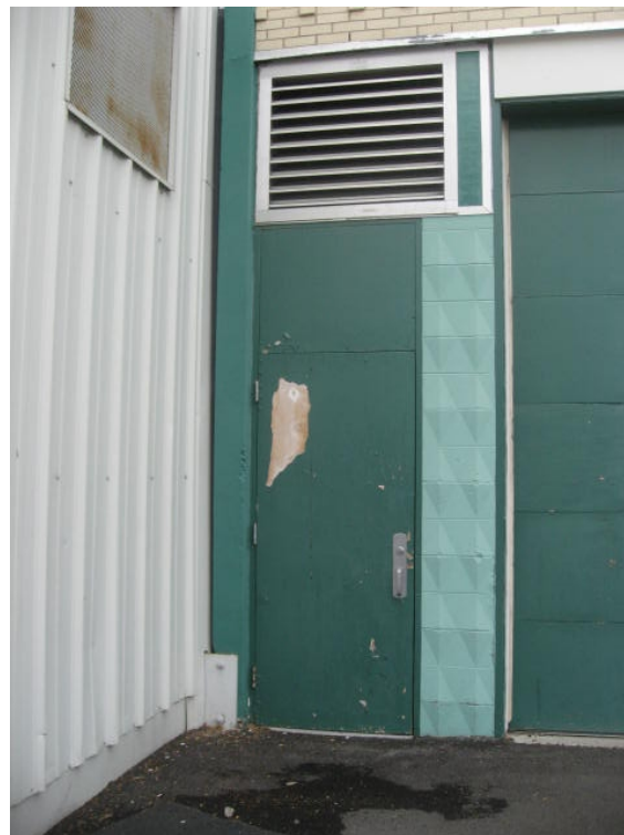
Typical deteriorated wood door in 1966 Section
