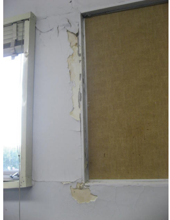
Water penetration on south wall.
