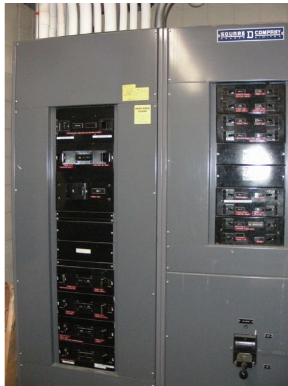
2000A, 120/208V Square D main switchboard.
