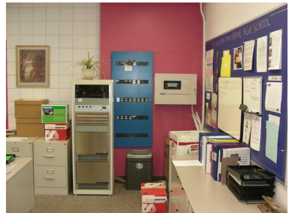
Pyrotronics System 3 fire alarm control panel in general office.
