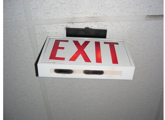
Incandescent exit sign.
