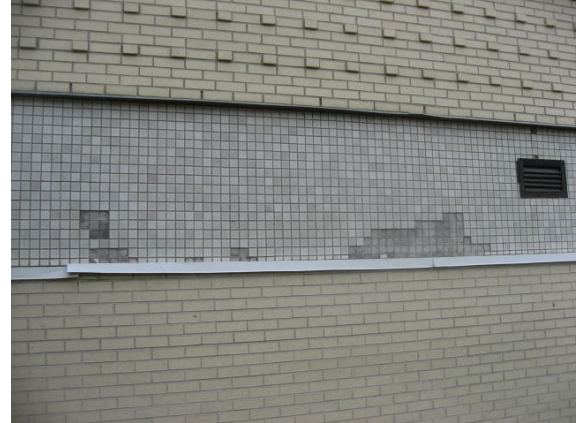
Missing tiles on west elevation of the 1983 Section.
