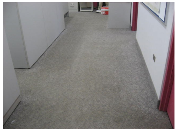
Worn carpeting typical throughout the office areas.
