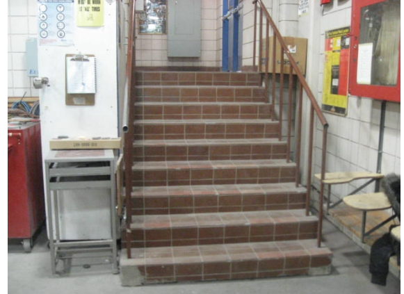
Cracked quarry tiles on stairs
