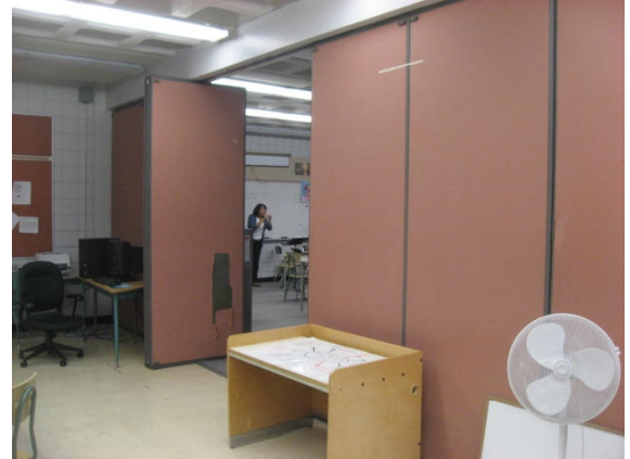
Damaged wall finish on folding partitions.
