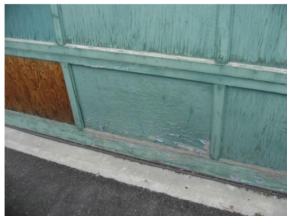
Deteriorated door panels in 1975 Building Construction Shop.
