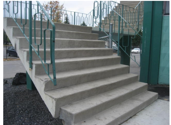
Uneven treads throughout stairs. Handrails not to current ABC code standards.
