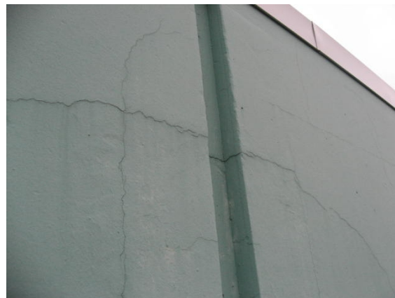
Cracked cement plaster walls on west wall - 1966 Section
