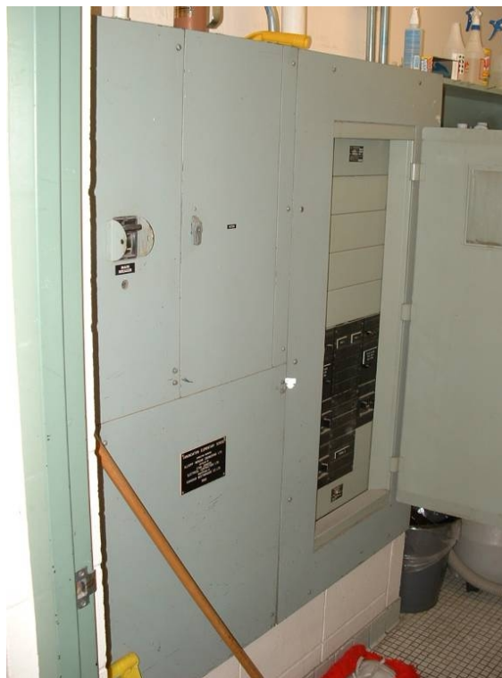
Main Westinghouse switchboard, 400A, 120/208V.
