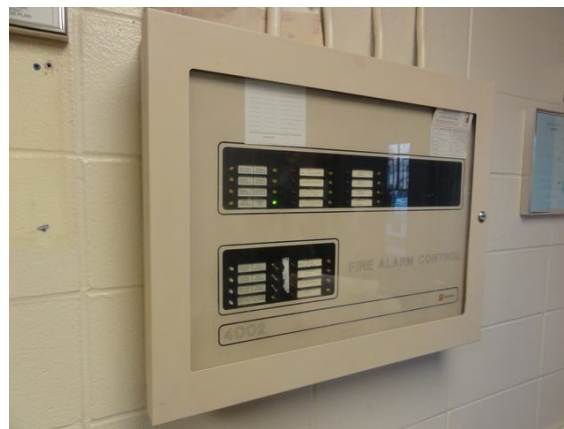
Simplex 4002 fire alarm control panel at main entrance.
