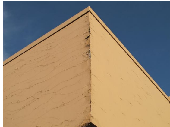
Damaged cement plaster finish at south-east corner of the 1969 Addition.
