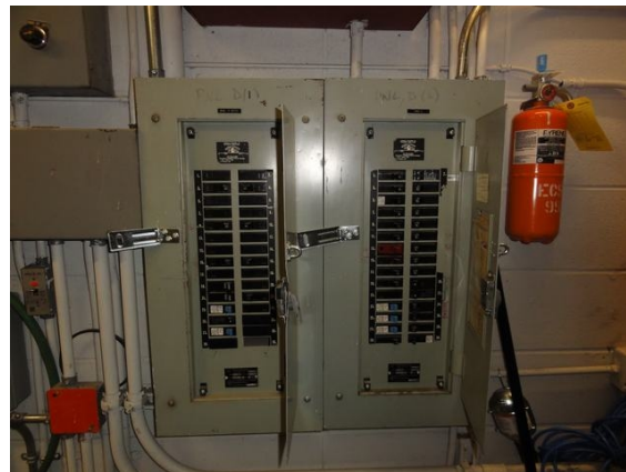
Aged Westinghouse branch circuit panels.
