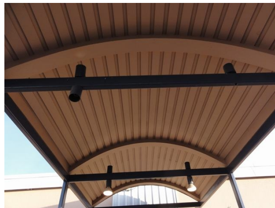
Incandescent lighting fixtures in entrance canopy.
