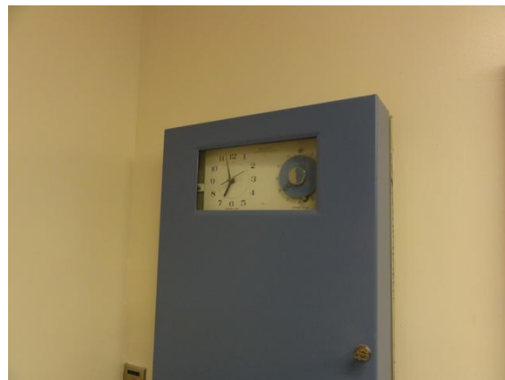
Obsolete Edwards clock system.
