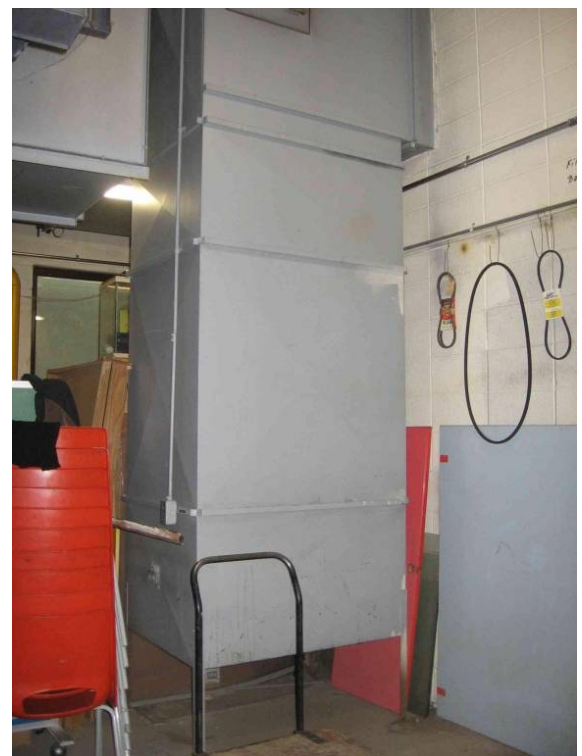
Combustion air duct outlet without baffle trap.
