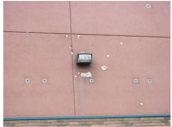
(1975) (East wall of Gymnasium 8) - has damaged stucco.
