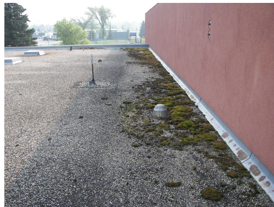
(1975) (North wall of Gymnasium 8) - has moss.
