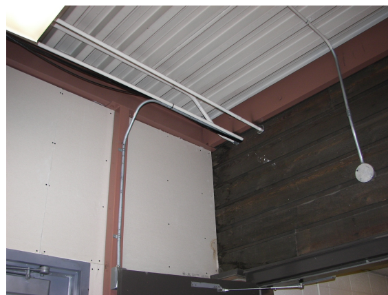
(1975) (Links to Portables 1975 and 1976) - have rotten wood siding above Corridor doors.
