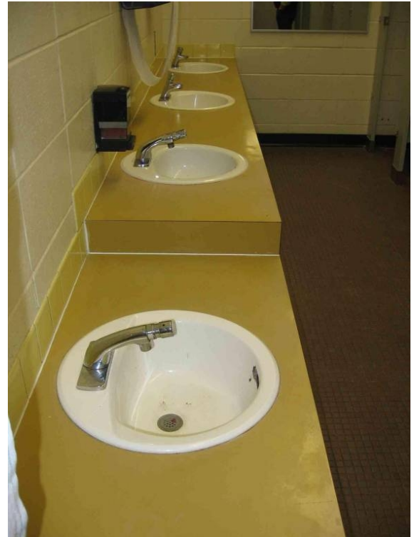
Lavatories are rusting at overflows. Porcelain has been chipped away, exposing rusting steel.
