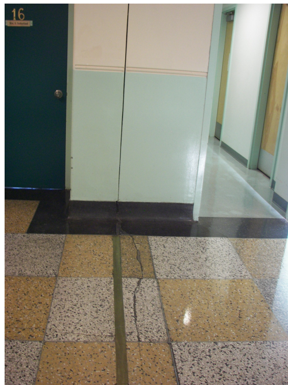
Areas between 1946 and 1950, 1946 and 1955 have cracked control joints.
