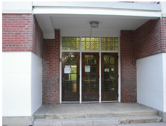
(1946) Original Building (Southeast Entrance) - has chipped steps.
