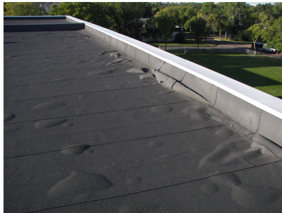
(1946) Original Building (west side) - has bubbles.
