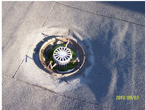
Roof drains have moss.
