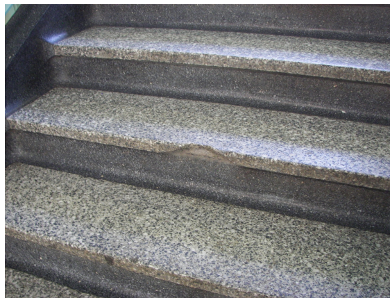
(1946) Original Building (Southeast Stair) - has damaged terrazzo stair finish.
