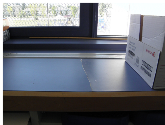
(1960) Addition (Second Floor - Classroom 33) - has damaged countertop.
