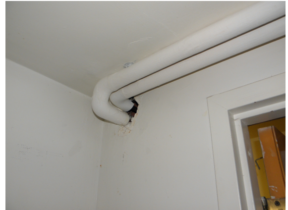
(1951) Original Building (Mechanical Room 16) - mechanical piping through wall need firestopping.
