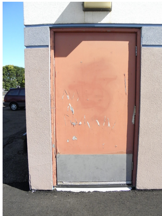
(1956) Addition (Main Floor - Corridor C9 Exit) - wood door and wood frame has worn out.
