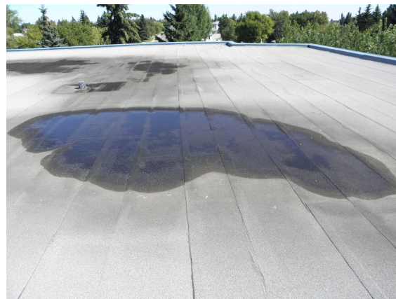
(1951) Original Building (Roof) - SBS roofing has ponding.
