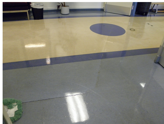
(1951) Original Building (Main Floor - Corridor C2) - has cracked sheet vinyl flooring.
