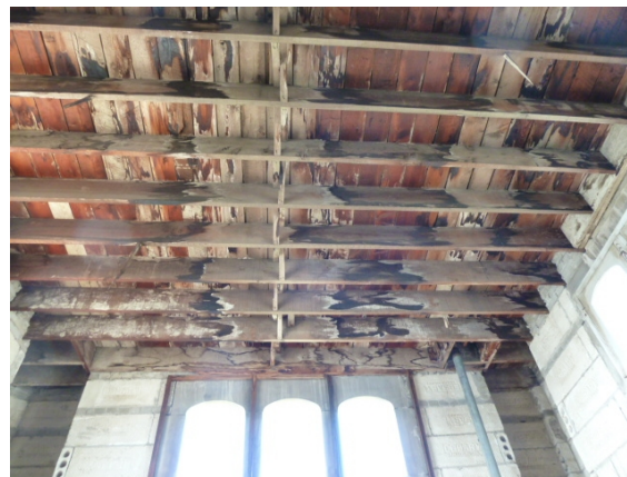
(1914) Original Building (Tower Roof) - has rotten roof wood deck and wood joists.
