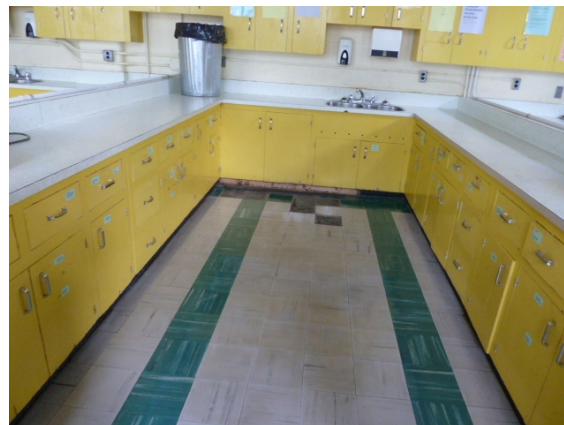
(1955) Annex (Home Economics 147) - has worn out vinyl asbestos tile flooring.
