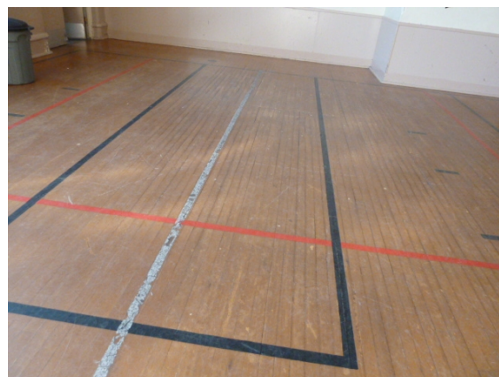
(1914) Original Building (Main Floor - Gymnasium 108) - has worn out wood strip flooring.
