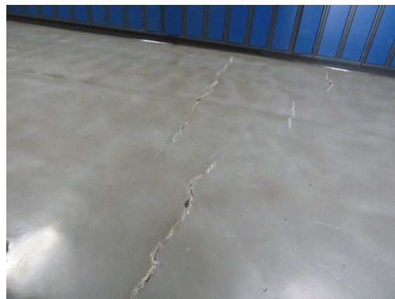
(1914) Original Building (Main Floor - Corridor C2) - has cracked linoleum flooring. (approx. 215 square metres)
