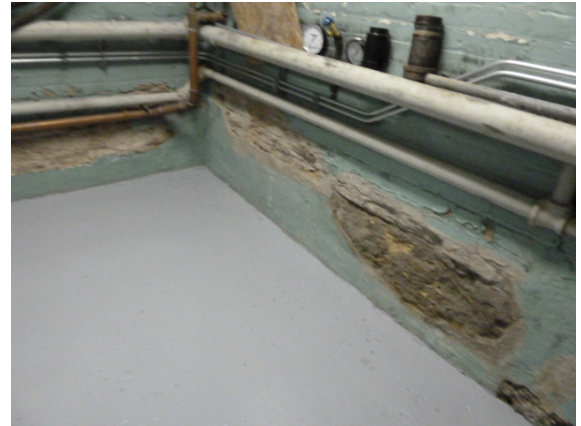
(1914) Original Building (Basement - Mechanical Room 1) - has damaged concrete foundation walls.
