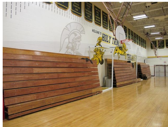
Re-tractable wood bleachers in gymnasium.
