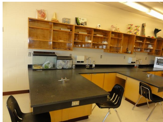
Receptacles within 1m of sink location are not GFI type.
