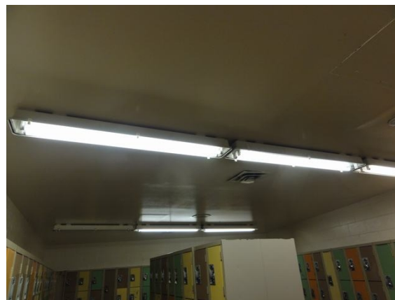
Lenses missing on fluorescent lighting fixtures.
