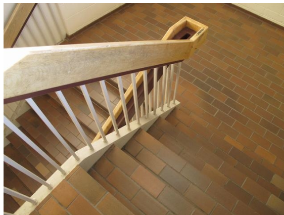
Deteriorated finish on wood handrail in all stairwells
