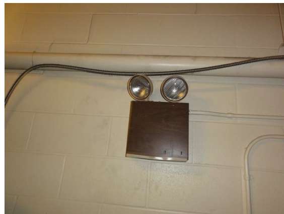
Aged emergency lighting battery unit in generator room.
