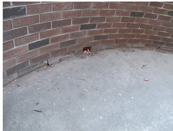
Movement of concrete slab opposite the west elevation of the school
