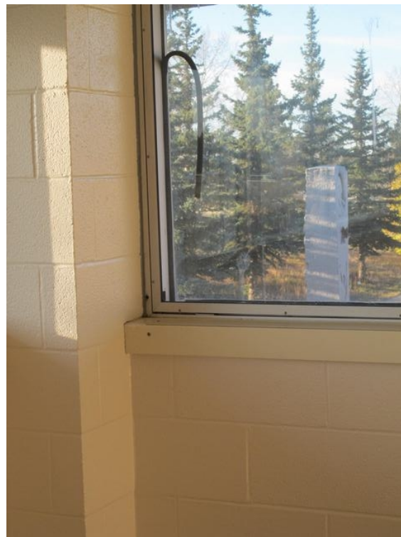
Failed window gasket observed in several locations
