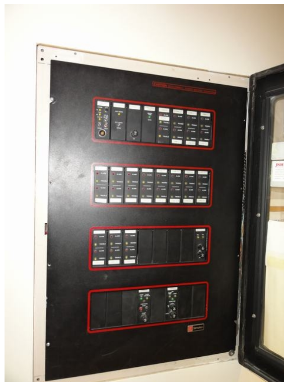
Aged Simplex 2100 fire alarm control panel in administration area.
