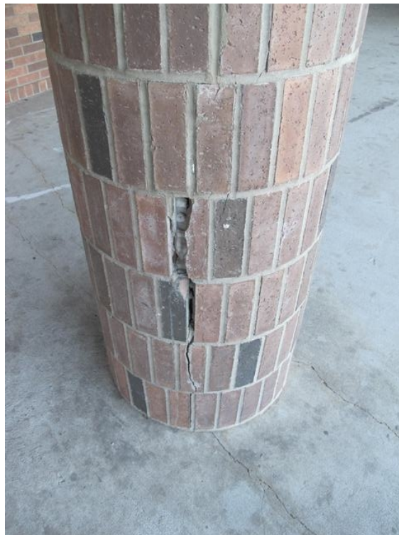
Cracked columns opposite the main entrance.
