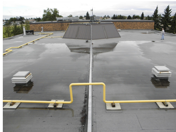
(1968) Original Building (Main Roof) - SBS roofing has ponding. (approx. 1000 square metres)
