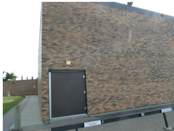
(1968) Original Building (Main Floor - Gymnasium 1) - has damaged wood doors and uneven hinges.
