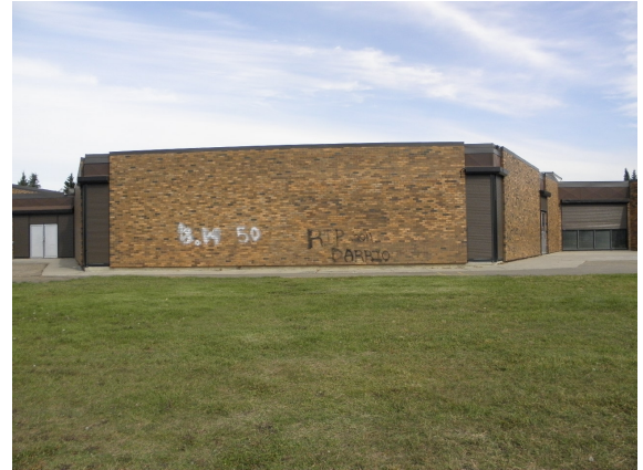
(1968) Original Building (Classroom 38, 39 - West side) - has graffiti on face brick
