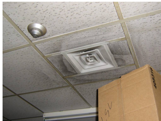
Dirty ceiling tiles.
