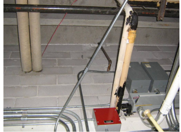
Cartier mechanical room, unsealed pipe penetrations
