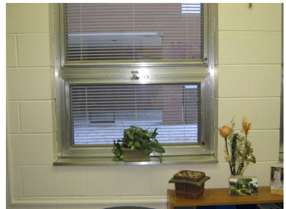
Window has loose weather stripping between window panes.
