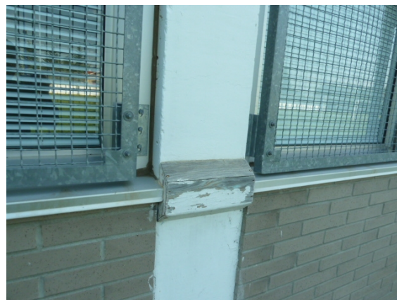
(1960) Original Building - has rotten wood trim and worn out paint.
