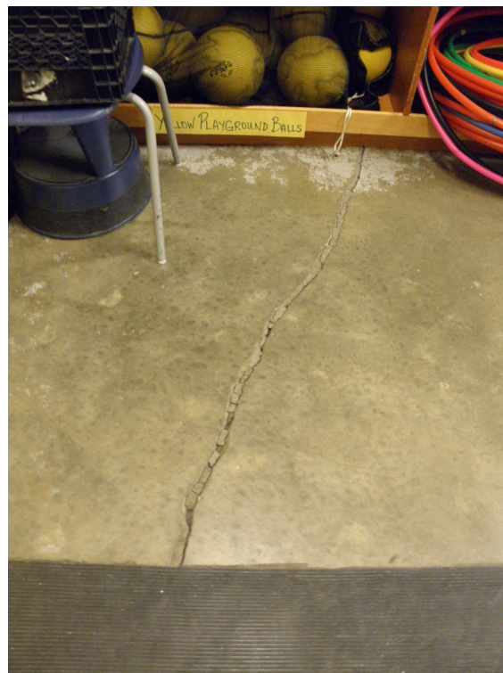
(1960) Original Building (Main Floor - Gym Storage 6) - has cracked concrete slab.
