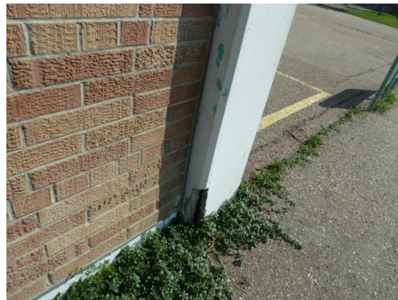
(1960) Original Building (Main Floor - Southeast corner) - has damaged cast in place concrete column.
