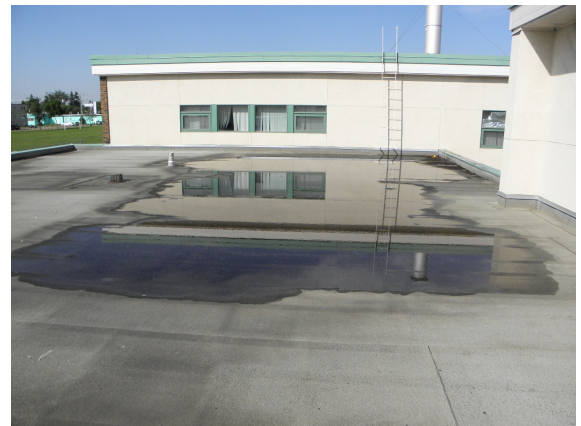
(1962) Addition (Low Roof) - SBS roofing has ponding.
