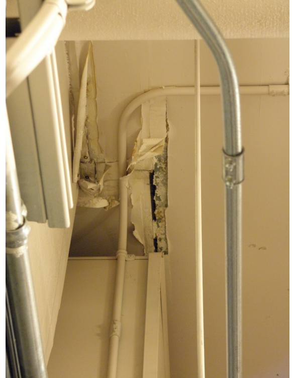
(1958) Original Building (Main Floor - Mechanical Room 35) - has damaged gypsum board ceiling finish.
