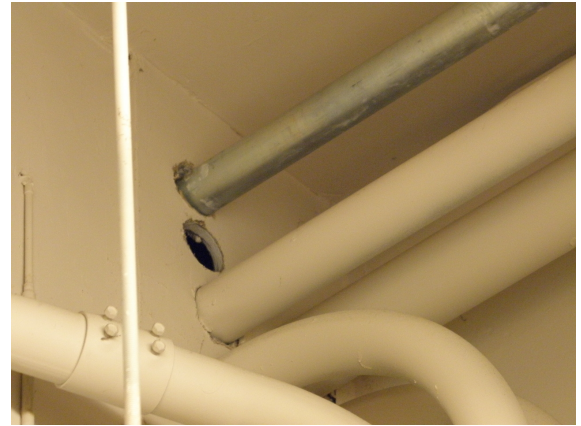
(1958) Original Building (Mechanical Room 35) - conduits penetrating walls need firestopping.
