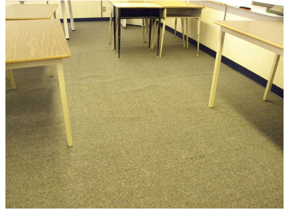
(1982) Addition (partial Classroom 42) - carpet flooring has ripples and open seams.
