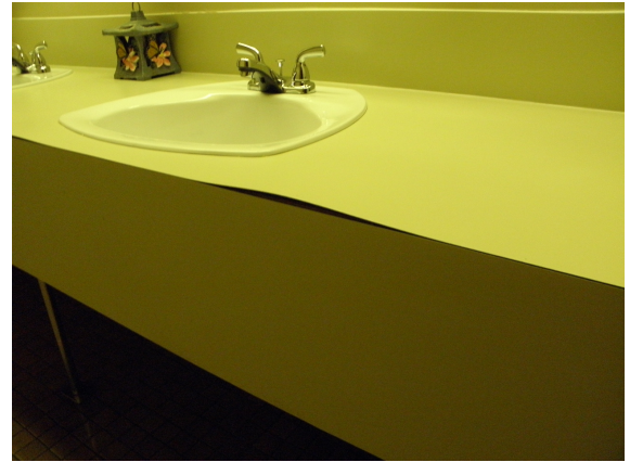
(1981) Original Building (Women's Washroom 26) - has damaged vanity.
