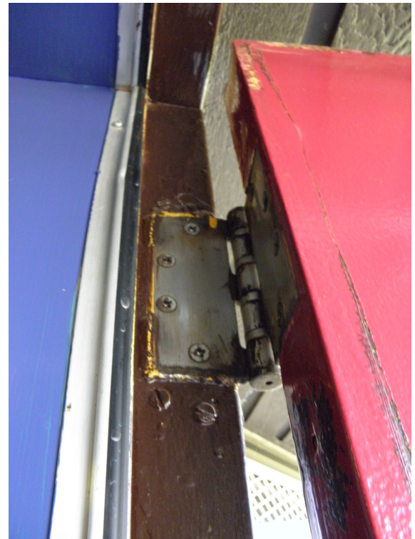
(1981) Original Building (Southwest Exit F2) - metal doors have welded hinges.
