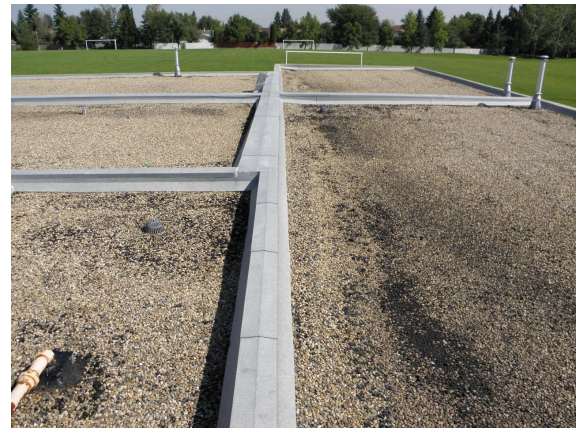
(1982) Addition - built-up roofing has blisters and bubbles. (approx. 410 square metres)
