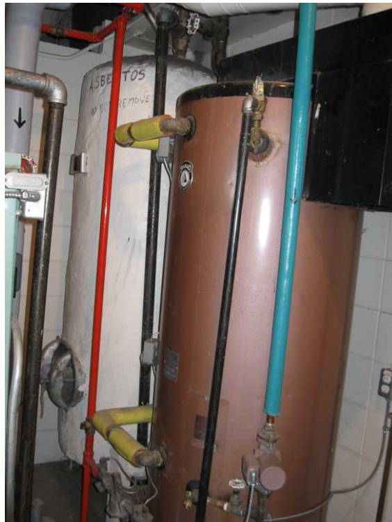
Domestic hot water heater and storage tank in Boiler Room
