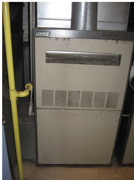
Typical gas fired furnace
