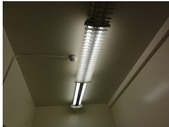
Louvered fluorescent T12 lighting.
