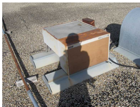
Old air cooled condensing unit on roof
