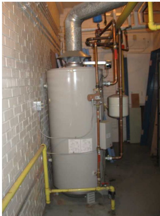
Uninsulated domestic water pipes in Mechanical Room #7
