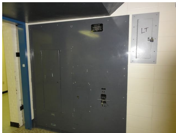
1200A main switchboard, located in corridor.
