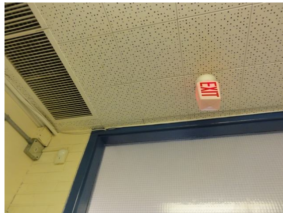
Exit sign is not code compliant.
