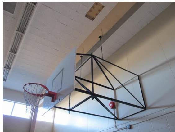
Missing ceiling tiles in the small gymnasium.
