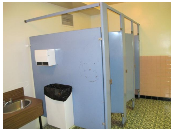
Damaged washroom partitions
