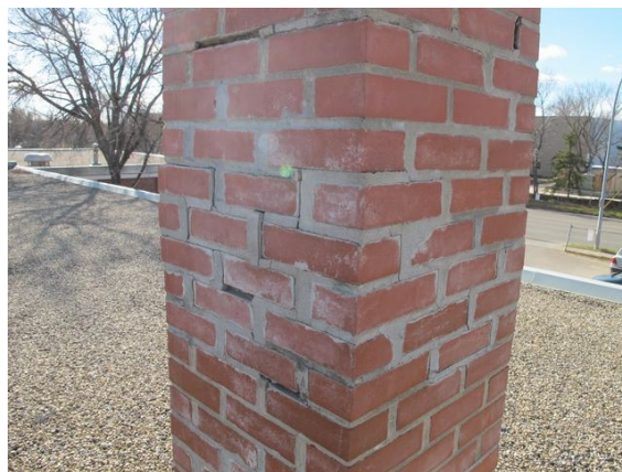
Deteriorated mortar on chimney - 1956 Section
