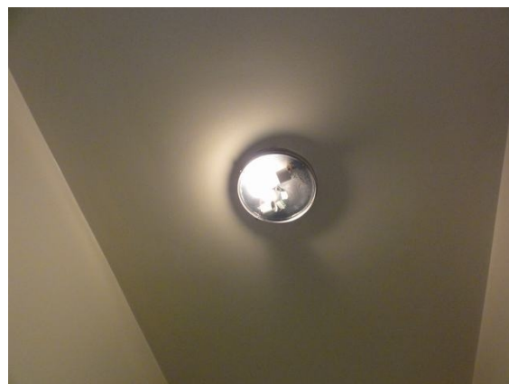
Incandescent fixture missing lamp housing.
