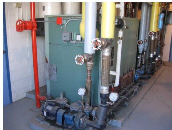
Hot water boilers in Boiler Room
