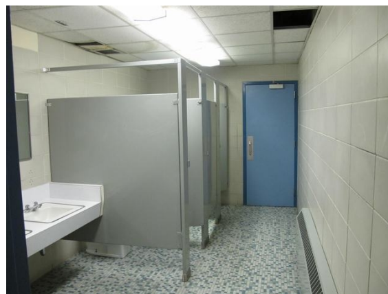
Stained and missing ceiling tiles in the washrooms.
