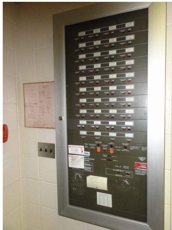
Edwards 6500 fire alarm control panel at main entrance.
