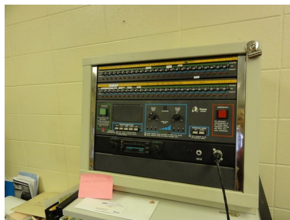
Obsolete Petcom 2200 P.A. System in general office.
