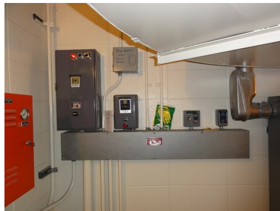
Aged motor starters in mechanical room.
