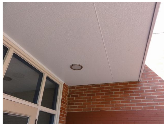
Recessed incandescent lighting installed in entrance canopy.
