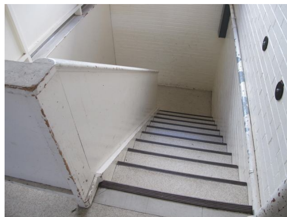
Deteriorated paint finish in the stair to the lounge area.
