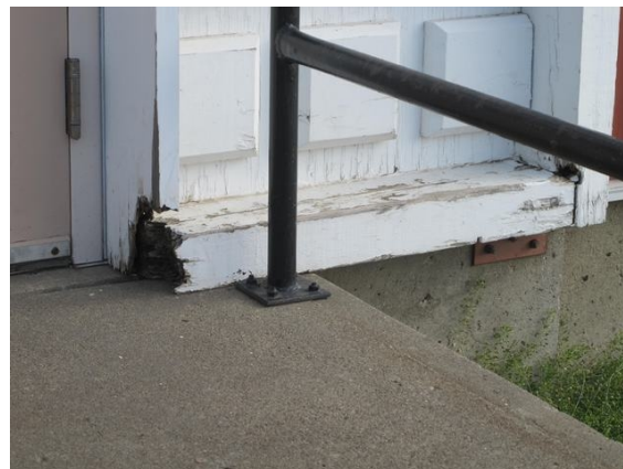
Deteriorated wood panels on 1974 Section - West elevation exit.
