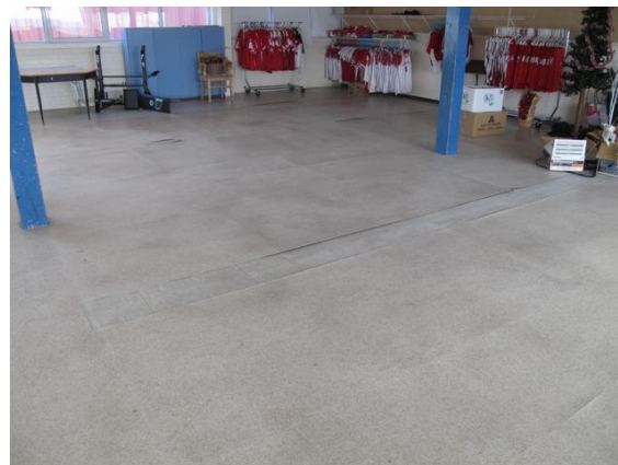
Deteriorated sheet vinyl in the 2nd floor lounge area.
