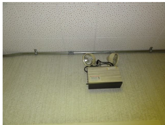
Aged emergency lighting battery unit.
