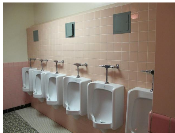
Stained grout between the ceramic tiles in the 1956 washrooms.
