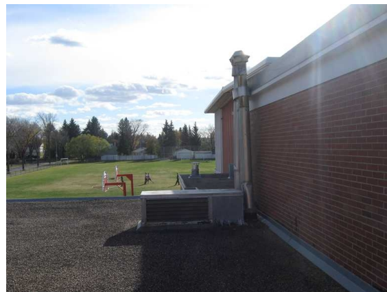
Three flue gas vents on roof from the furnaces in Mechanical Room #4
