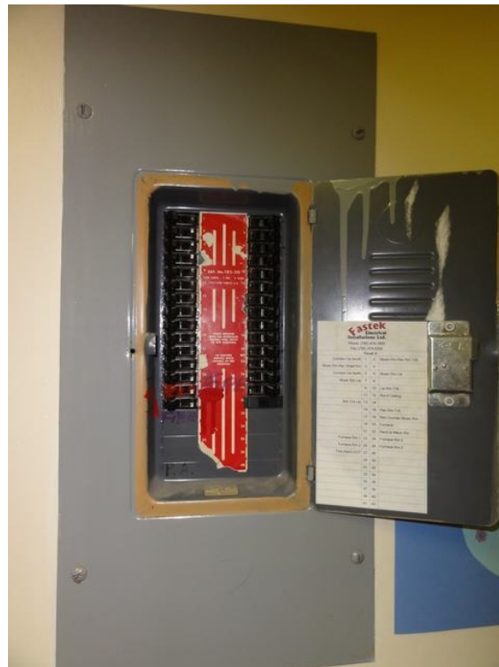
Federal Electric 120/240 branch circuit panel.
