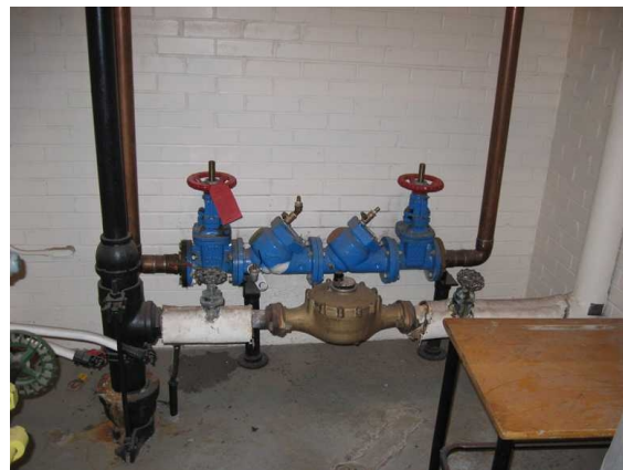
Domestic water meter with backflow preventor for standpipe system only.
