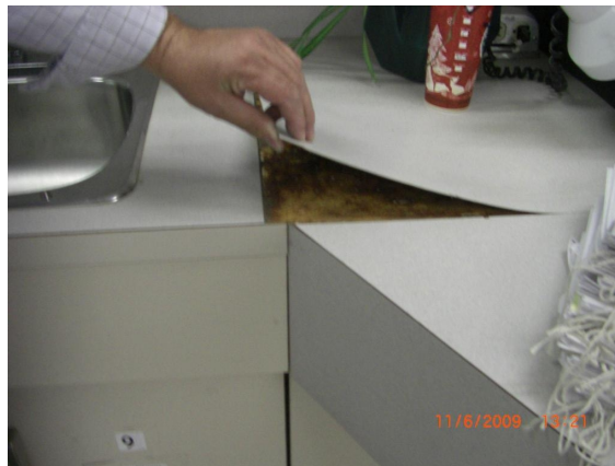
(1971) Addition Science 134) - has damaged countertops.
