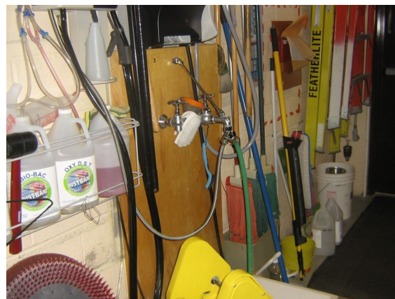
Service Sink in Mechanical Room.
