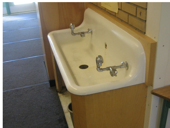
Double Bubbler drinking fountain is rusting.
