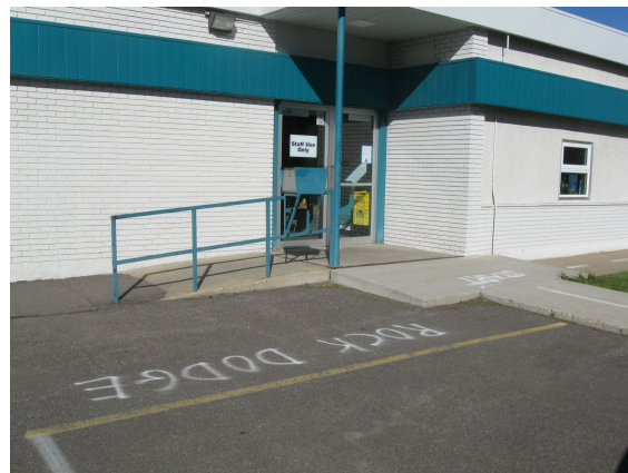
Ramp does not have a railing on both sides. No wheel guard at bottom of existing rail.
