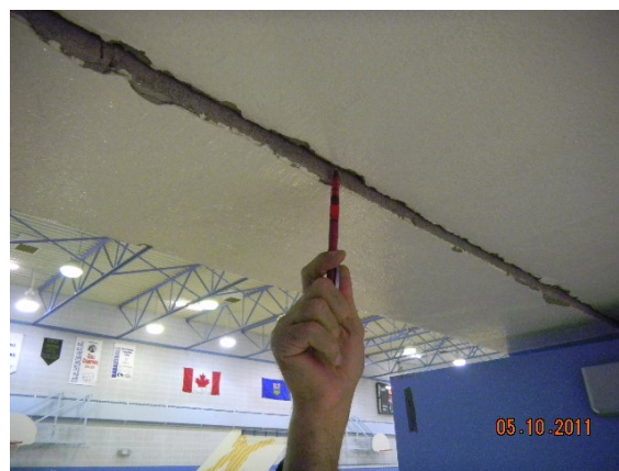
NW corner of 1992 addition has settling issues at link between the two gyms
