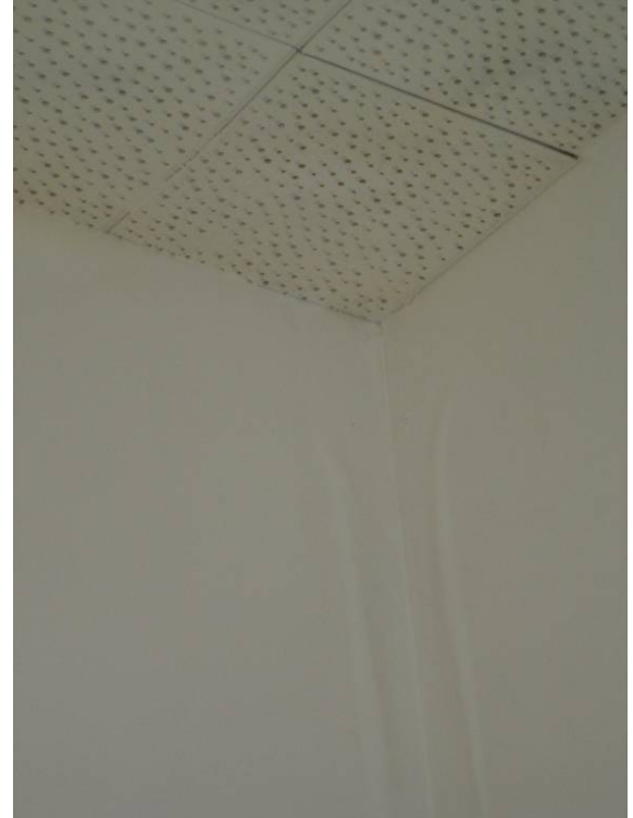
Ceiling tile sagging.
