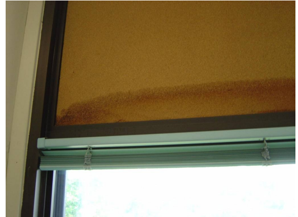
Moisture staining on interior cork surface.
