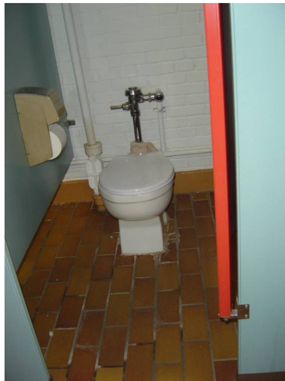
Poor grout tile joints in washroom
