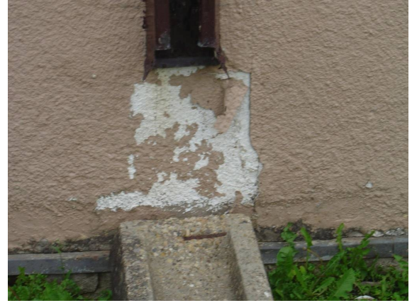
Paint finish peeling below downspouts.
