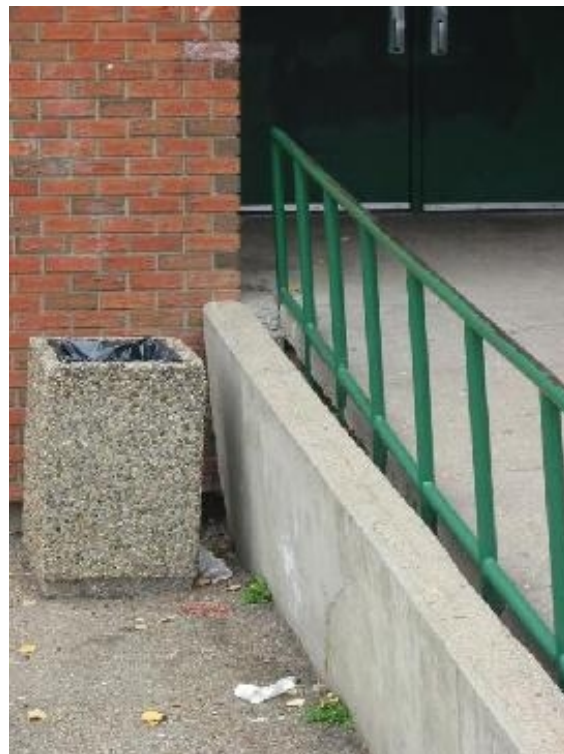
Failure at retaining wall ramp. Handrail too low.
