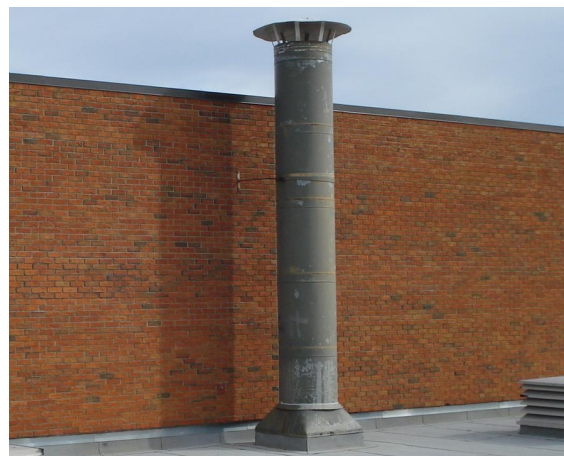
Rust on the exterior portion of the boiler chimney.
