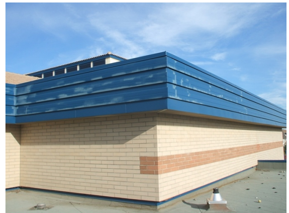
Metal siding showing oxidization taken from the SW roof level.
