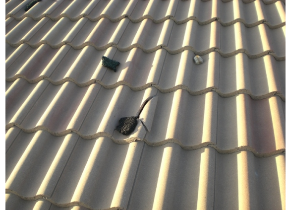
One of the areas with crack roof tiles
