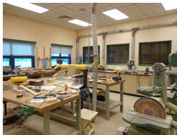
Dust collection outlets in wood working room.
