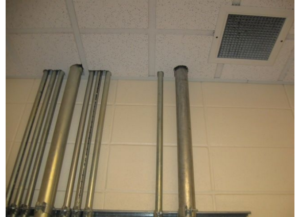
Firestopping missing where conduits pierce ceiling tiles.
