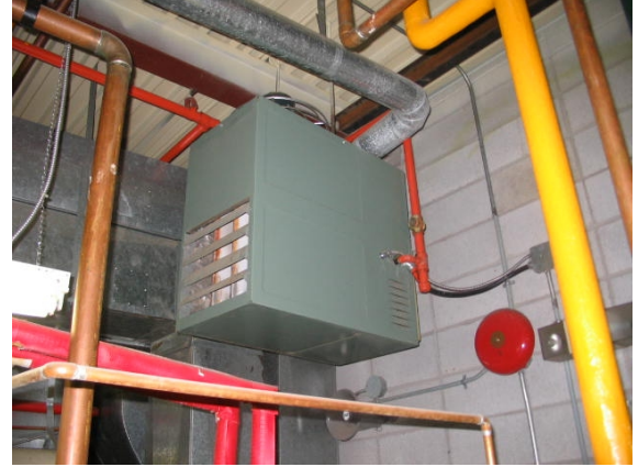
Unit Heater in Mechanical Room.
