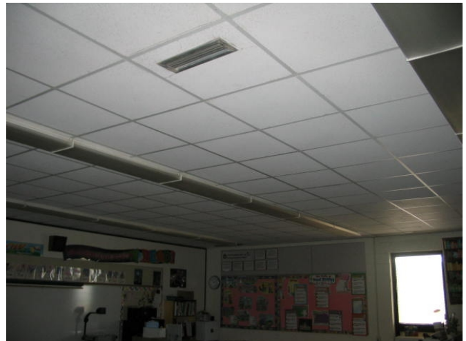
Supply air grille in classroom.
