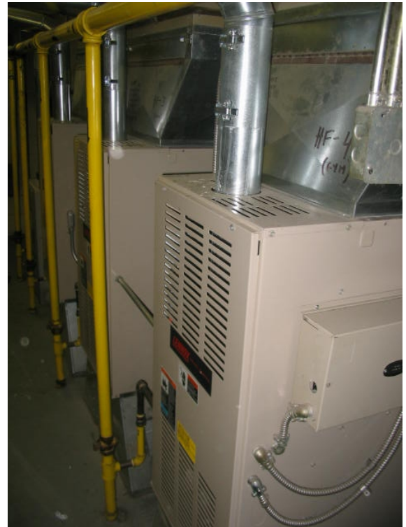
Furnaces serving Gymnasium.
